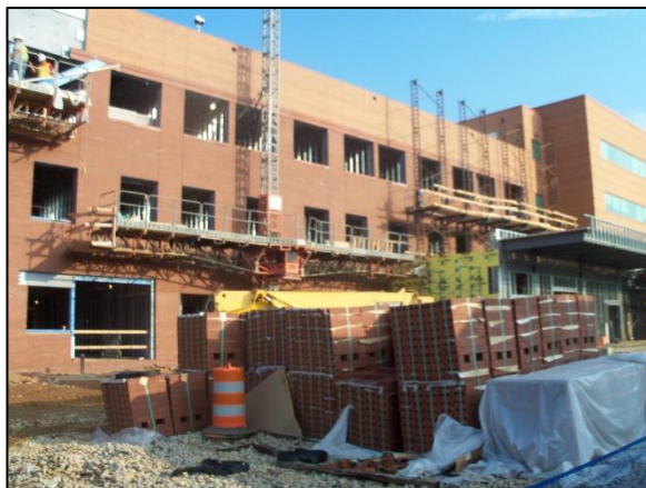
Figure 9 - Fraco Lifts which didn't allow work to be done underneath along with large amounts of brick taking up valuable laydown space for an extended period of time can be seen here. Personal photo taken by Chris Pozza.
