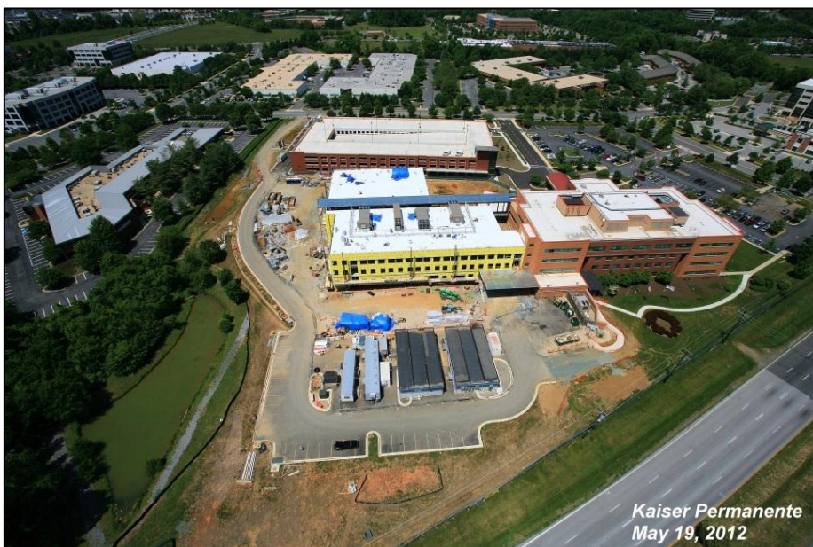
Figure 1 - The stormwater management pond protection can be seen in the lower left of the image. This area has been protected throughout construction and the pond will be completely restored upon completion of the project. Image courtesy of DPR Construction.
