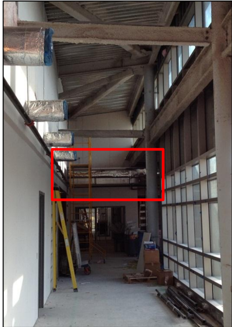
Figure 8 - View of corridor space in Area B on the third floor looking south. Ductwork can be seen crossing this space running from Area B to Area C along with the clerestory window in the upper right of the image. Personal photograph taken by Chris Pozza.
